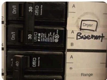
Dryer breaker in the panel
