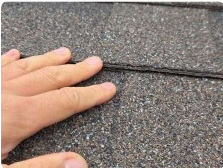
Raised area at a fastener, front side
