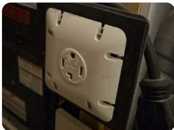
Dryer unplugged at the outlet
