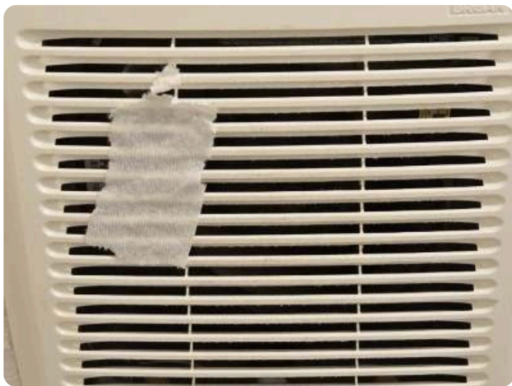
Dust on the upper bathroom fan
