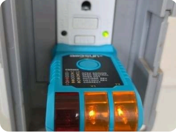
Exterior GFCI outlet tested
