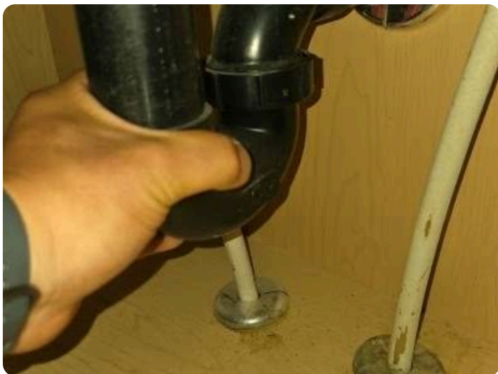
Dry drain trap under a sink
