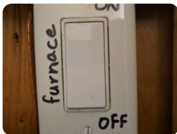
Furnace shut-off switch
