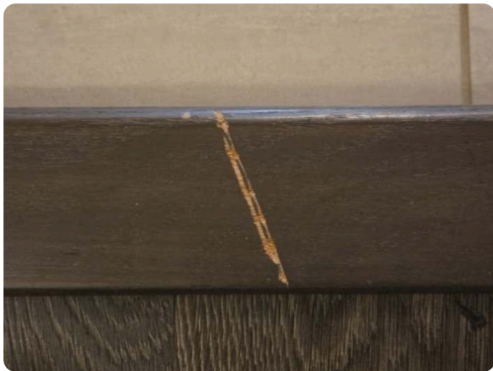
Damage at the stair edge
