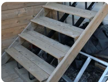
Deck stairs without a handrail
