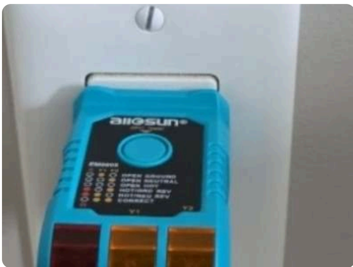
Outlet tester showing no power
