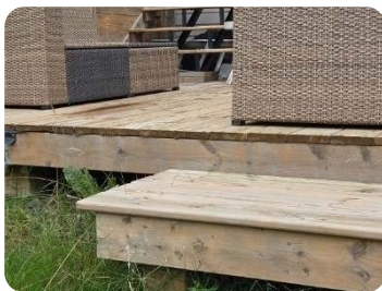
Deck without guards along its open side
